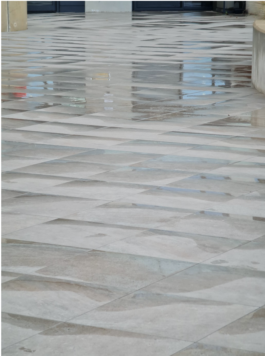
Photograph 5. Depicts water retention on a podium tile installation during the morning at 10 am after a night of rain.
