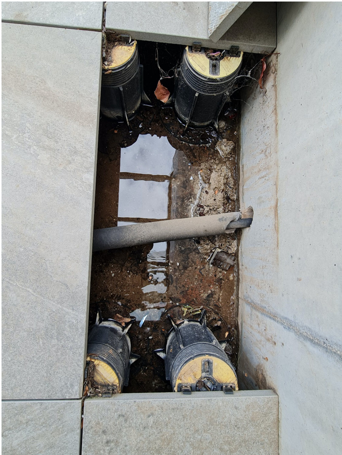
Photograph 11. shows water retention beneath the tiles due to insufficient gradients.
