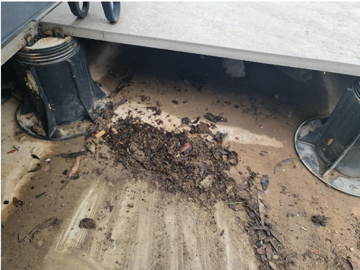
Photograph 4. depicts debris under a podium system 2 years after installation.
