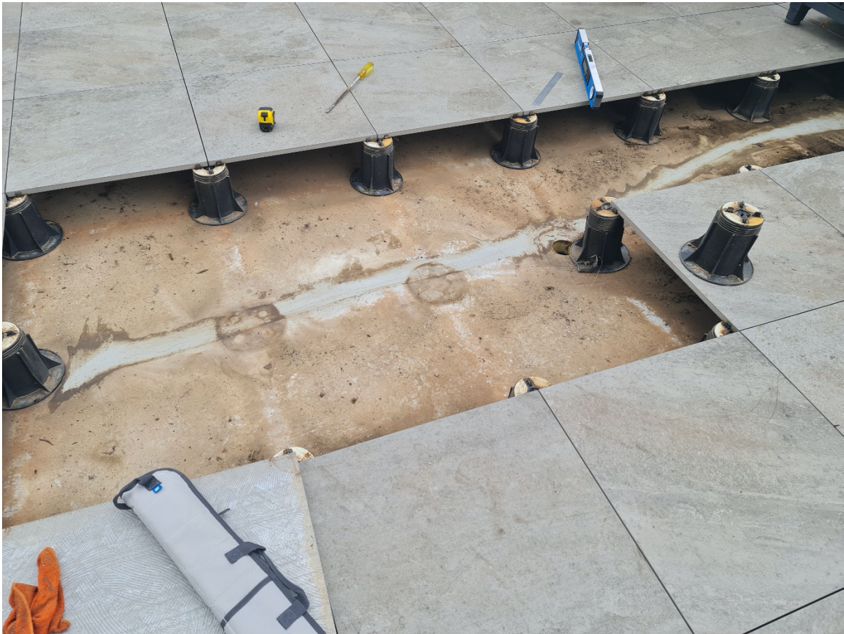
Photograph 7. shows dirt and debris accumulated on the waterproofing membrane beneath the tiles after approximately 2 years. In this image, the dirt was cleaned off the membrane to examine a failure in the membrane beneath.
