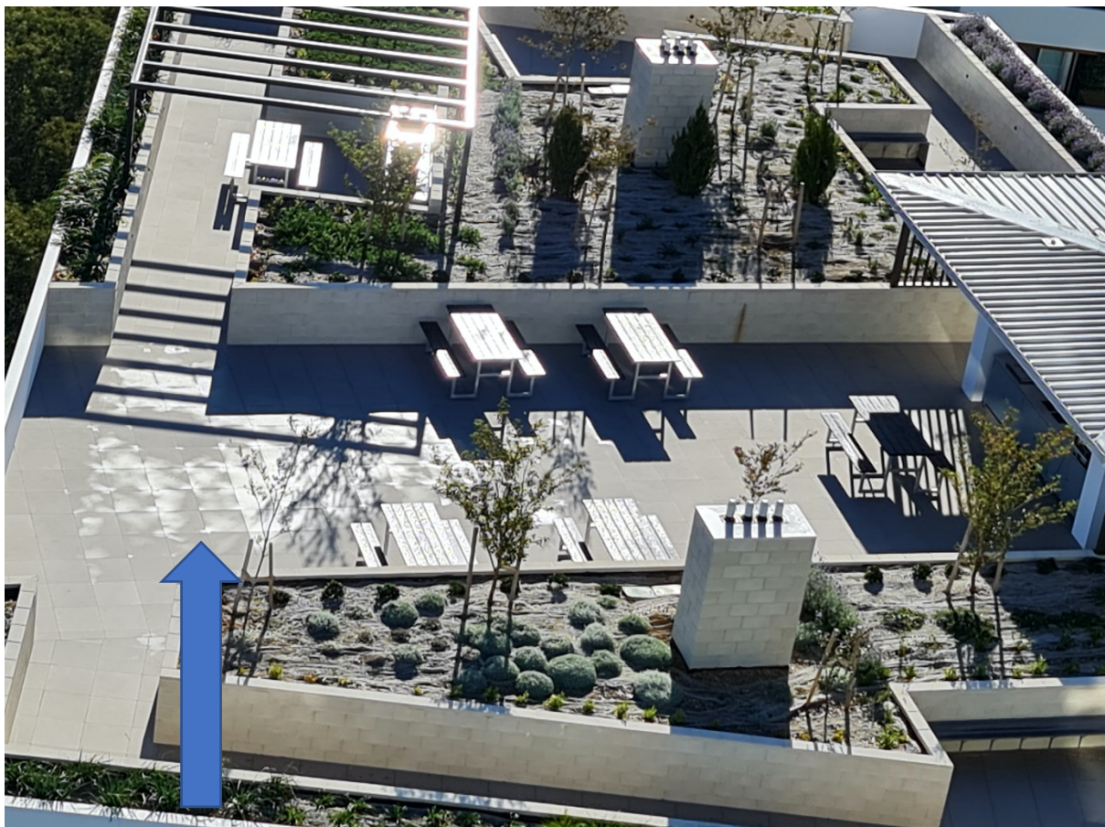
Photograph 6. depicts water retention on the surface of a podium tile installation.
