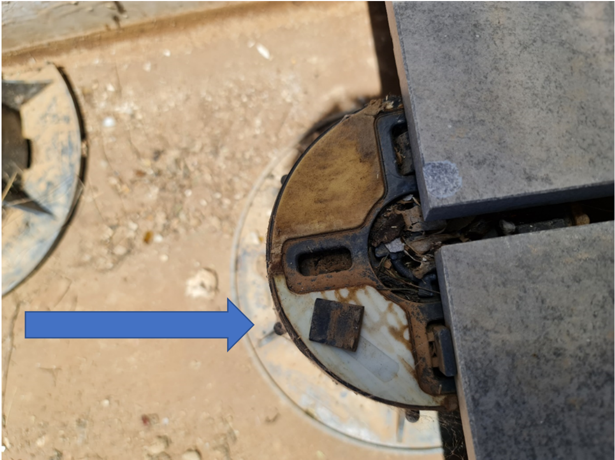
Photograph 9. shows broken spacer lug
