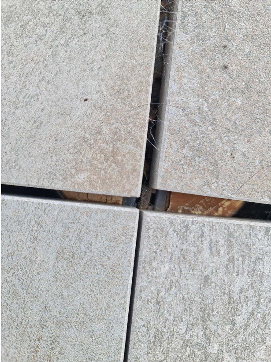
Photograph 10. shows missing spacer lugs
