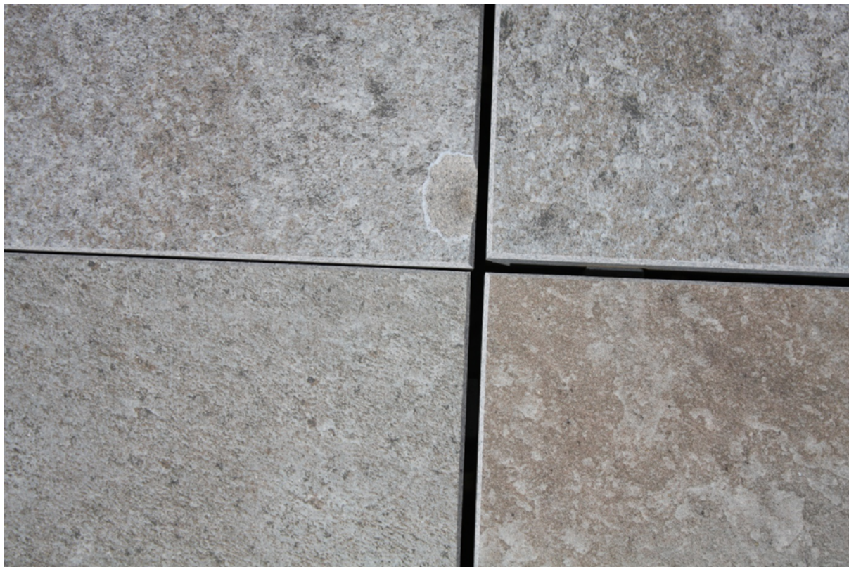
Photograph 8. shows chipped tile from differential movement.
