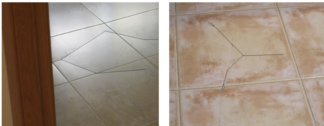
Figure 13. Cracks tending to form angles of 120^\circ .
