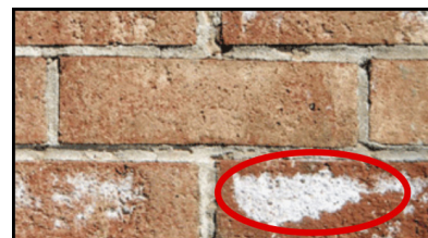
Figure 5. Efflorescence in a brick.
