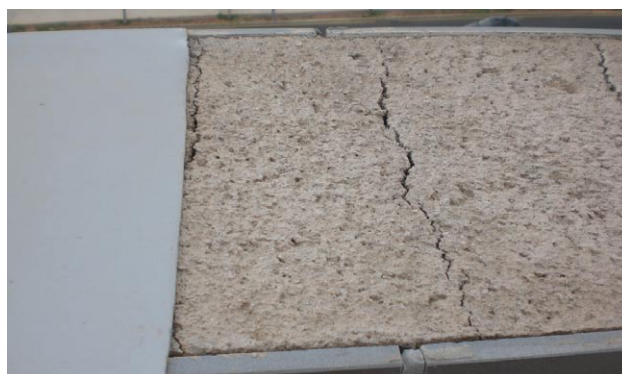
Fig. 1-Absence of Coping on a Terrace Wall
