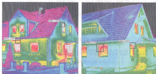
Figure 2. Thermographic images of a house before and after reform.
