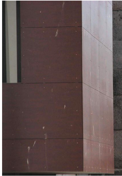
Figure 6. Panels made of wood-based materials are being increasingly used in contemporary Portuguese architecture, despite certain inconveniences after some years of exposure to climate aggressions. Overall, ceramic materials respond better to these problems and can be the better alternative in ventilated façades.
