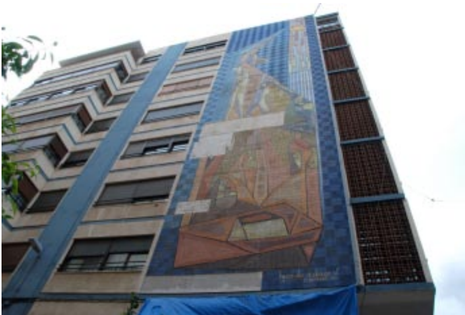
Figure 15. Beginning of the restoration work. Removal of pieces, from the bottom up.
