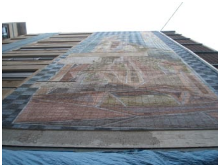
Figure 13. Beginning of the restoration work, from the bottom up, to avoid detachments.
