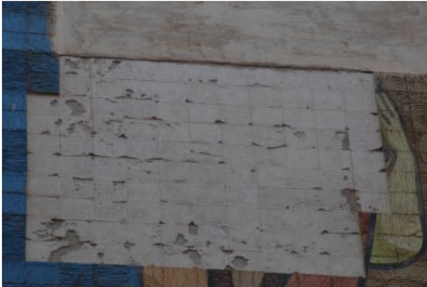
Figure 16. Surface state of the mural before the restoration work.
