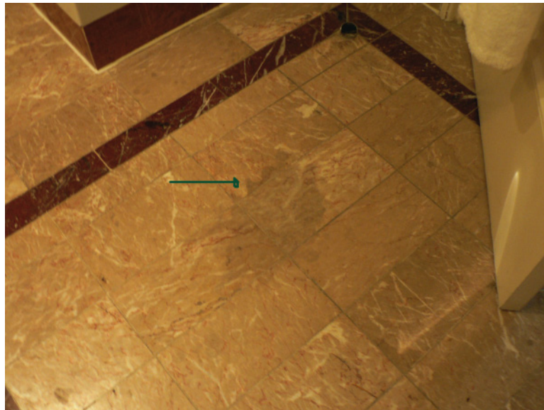
Figure 7. Natural marble in a luxury hotel London, England is stained with red wine. Porous stone that requires annual sealing offers minimal stain resistance in either residential or commercial settings. A rectified quality ceramic tile is virtually indistinguishable from the natural stone and therefore provides the aesthetic cachet in addition to superior technical properties.
