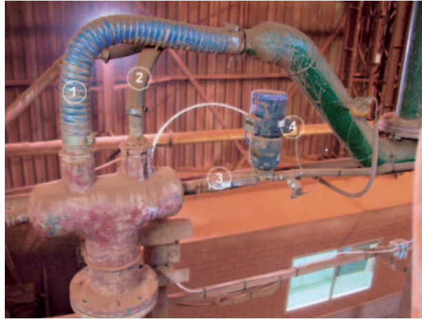
Figure 5. Detail of water and deflocculant feed to the mill
