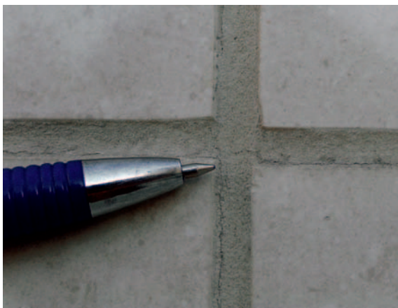
Figure 12. Small cracks between grouted joint and porcelain tiles edges that happened in many facades that have been inspected during the field survey.
