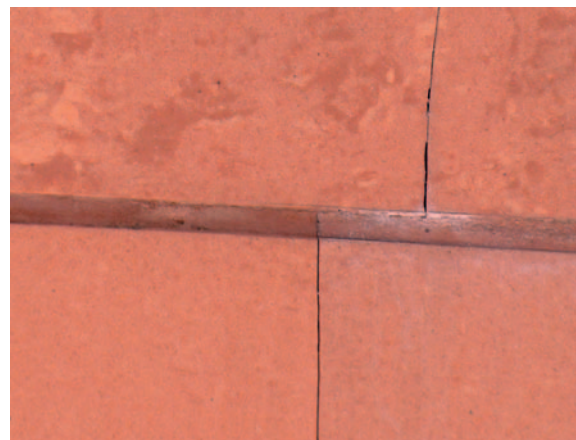
Figure 13. Example of crack observed where wire anchorages were attached to the back of tiles in order to improve bond stability.
