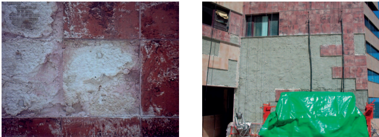
Figure 14. Severe bond defects occurred in two cases. After six years tile facade was entirely repaired.
