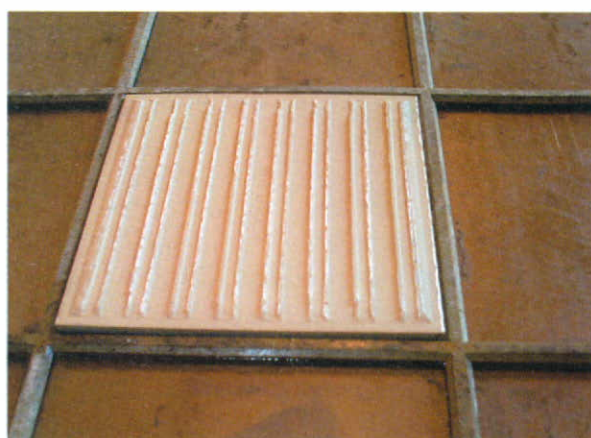
Figure 14 - Close-up view of tile bonding surfac.
