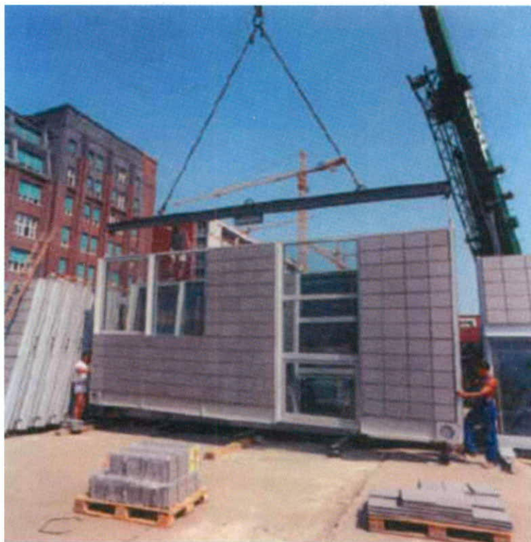
Figure 22 - Full story-height prefabricated tile panel integral with windows.
