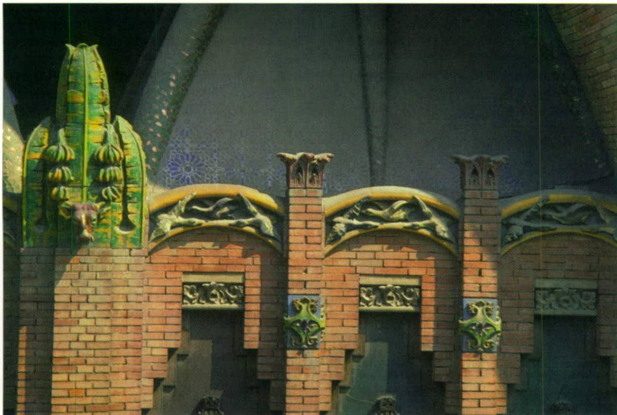
Outside detail of the Colon Market, currently awaiting restoration.
