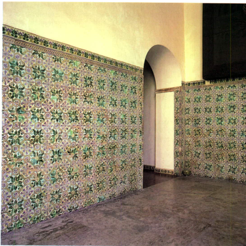
Tile skirting in the schoolyard of the Colegio del Corpus Christi in Valencia, a XVIth century building with serious preservation problems.
