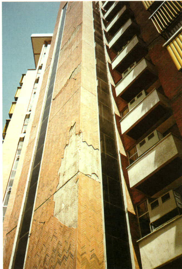
Figure 2. General failure of ceramic tile façade. Extruded stoneware were used with an ordinary mortar. Weather conditions during summer are very severe. Temperature above 40°C is usual. Control joints were built after the bond had failed.
